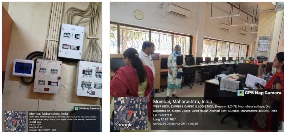
Plate 1: Assessment of the energy and electrical areas
